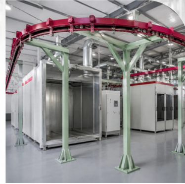
Enclosed Track Conveyor
